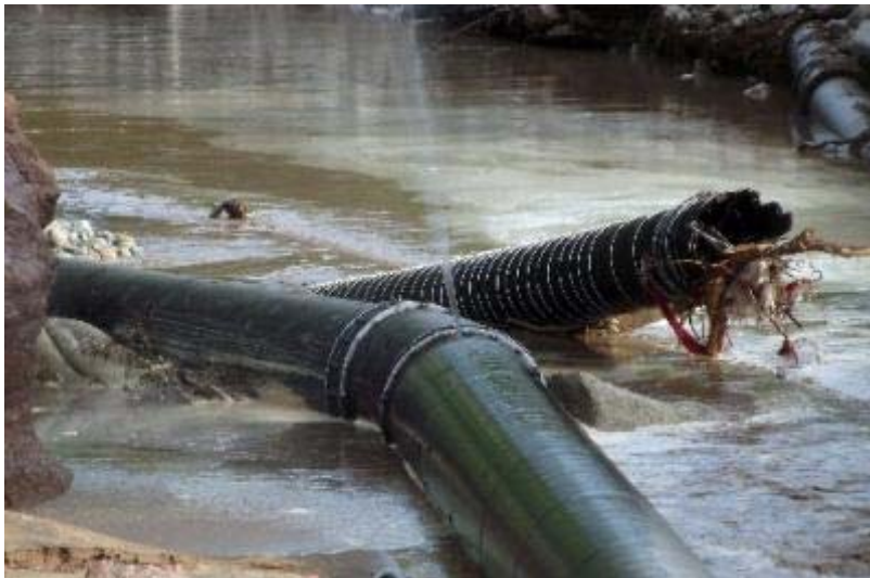
Last month's flood exposed water transmission lines near the city of Loveland's Water Treatment Plant. This 48-inch line survived with minimal
