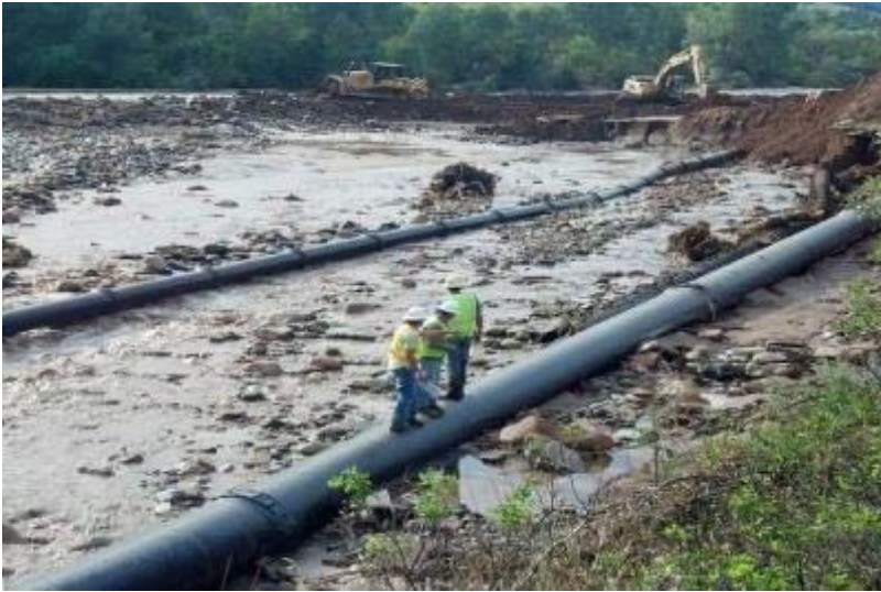
Following completion of an unprecedented project to divert the flooded Big Thompson River last month, city workers evaluate a 48-inch water transmission
